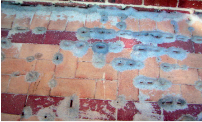
Paving undermined by big-headed ants
