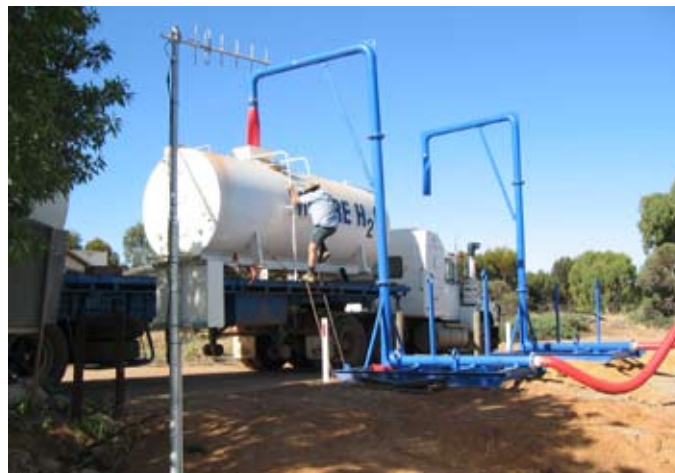
Bruce Sayer, a local water carting contractor picking up a tanker load from the Merredin desalination plant
