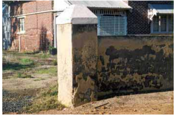
Salinity damage to a garden wall
